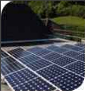
Solar photovoltaic (PV)
