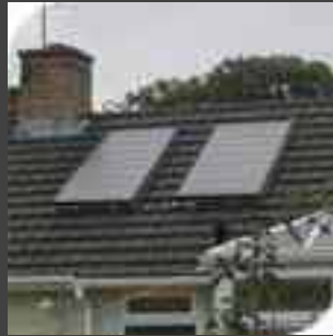
Solar thermal hot water
